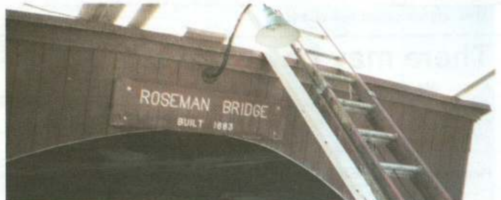
One of the bridges that will appear prominently in the upcoming movie, "The Bridges of Madison County," was being "aged" in preparation for the cameras.
